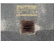
Point 2: Drainage System with catch basin. No large rocks to block flow.
