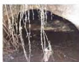
Point 2 shows the drainage pipe blockage at the Freetown Boat Ramp at #11.
