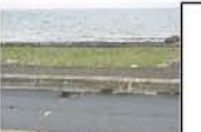
POINT 3 PHOTO: Catch basin on causeway and concrete road. Catch basin is closed.
