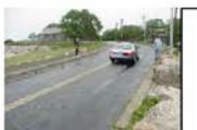
POINT 2 PHOTO: Catch basin on causeway and concrete road. Catch basin is closed.
